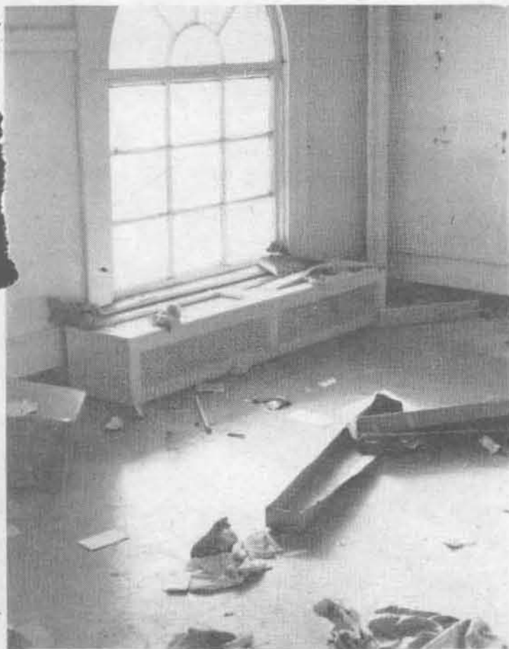
THE PARTY'S OVER: A room in the old Administration Building shows the remains of organization moves to other parts of the campus. The building is currently scheduled to be demolished soon. [Photo by Jeanne Vogel-Franzl].
